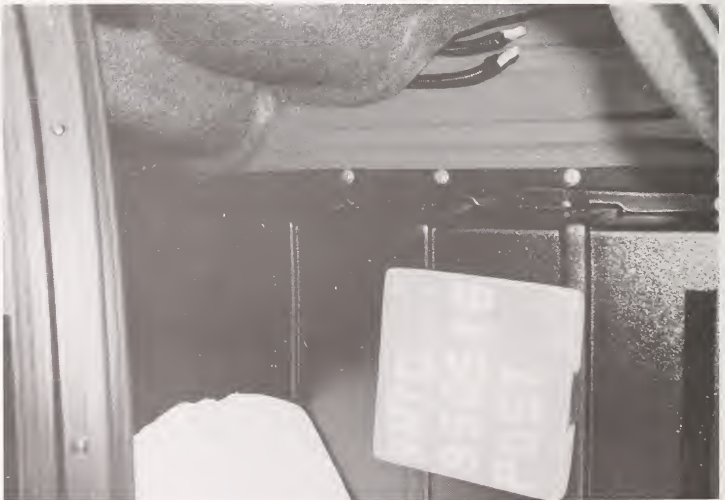
Figure A-31 Post-test Rear Battery Box Cover - View 2
